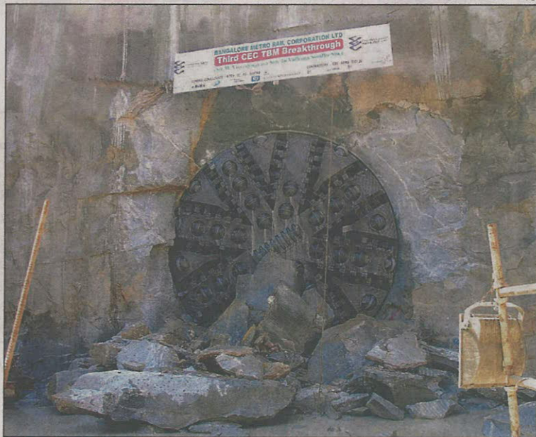
SHE FINALLY ARRIVES: Helen has been burrowing 60 feet under for the underground section of Metro's eastern line between Majestic and Minsk Square
